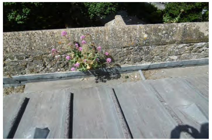
VEGETATION GROWTH IN THE NORTH AISLE PARAPET
