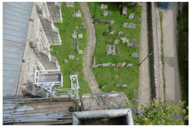
VEGETATION GROWTH IN THE TOWER BUTTRESSES
