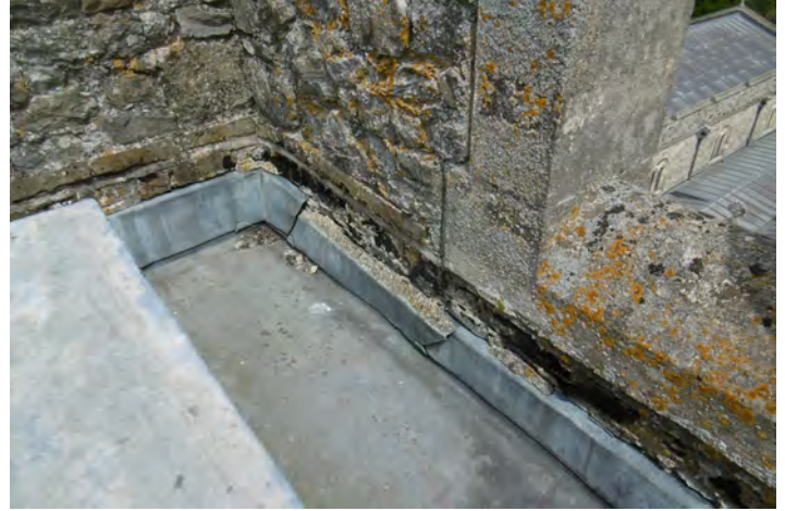
DECAY OF THE TOWER ROOF ABUTMENT FLASHINGS
