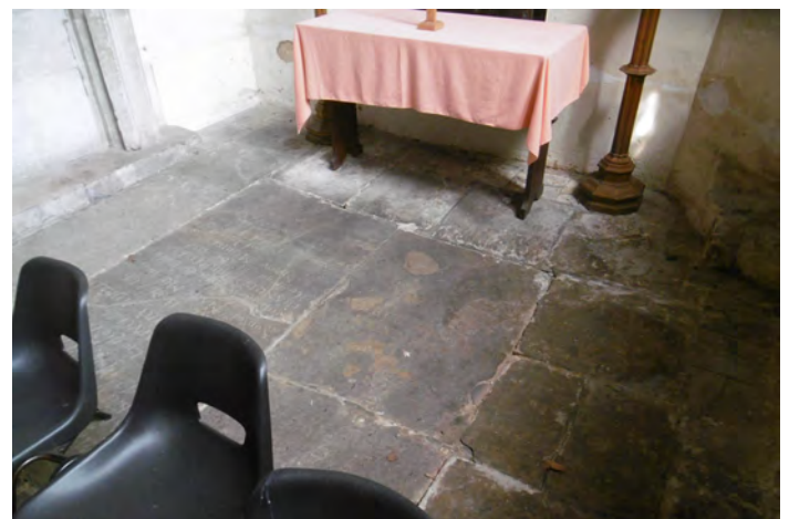
SETTLEMENT IN THE SOUTH CHANCEL AISLE
