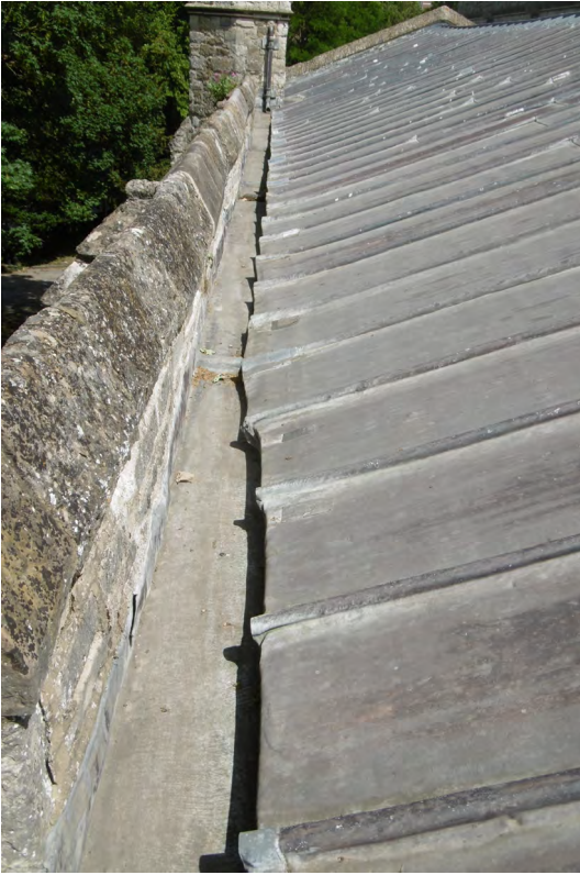
LEAD SLIPPAGE ON THE NORTH SLOPE OF THE NORTH AISLE
