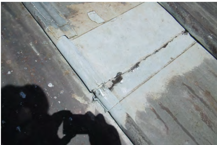
LEAD SLIPPAGE ON THE EASTERN NAVE ROOF
