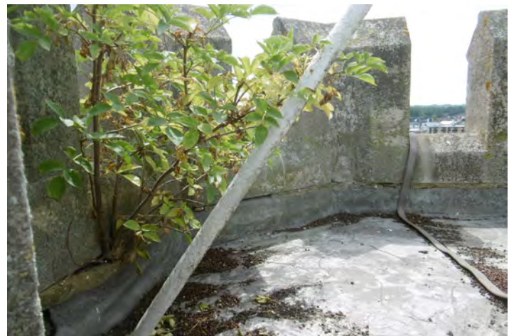
VEGETATION GROWTH ON THE TOWER TURRET ROOF
