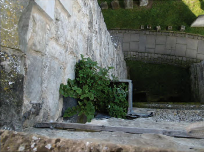
BLOCKED DOWNPIPE TO THE SOUTH AISLE
