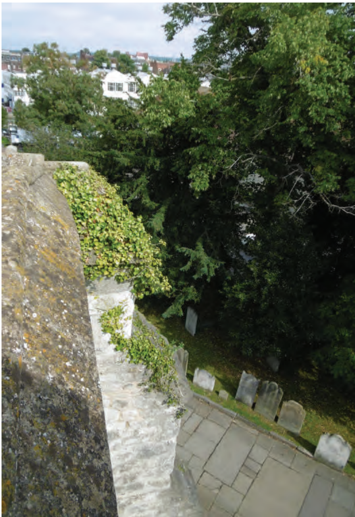
PLANT GROWTH ON THE EAST GABLE
