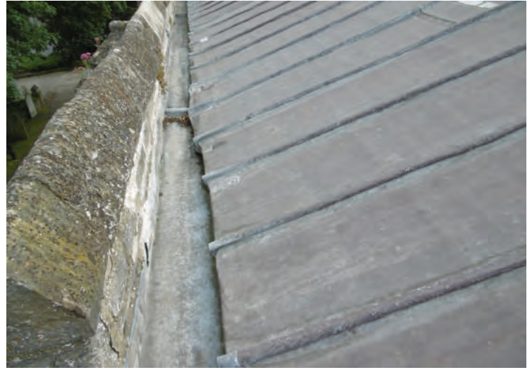
LEAD CREEP ON THE NORTH AISLE ROOF
