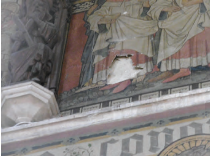
DETERIORATION OF THE WALL PAINTINGS
