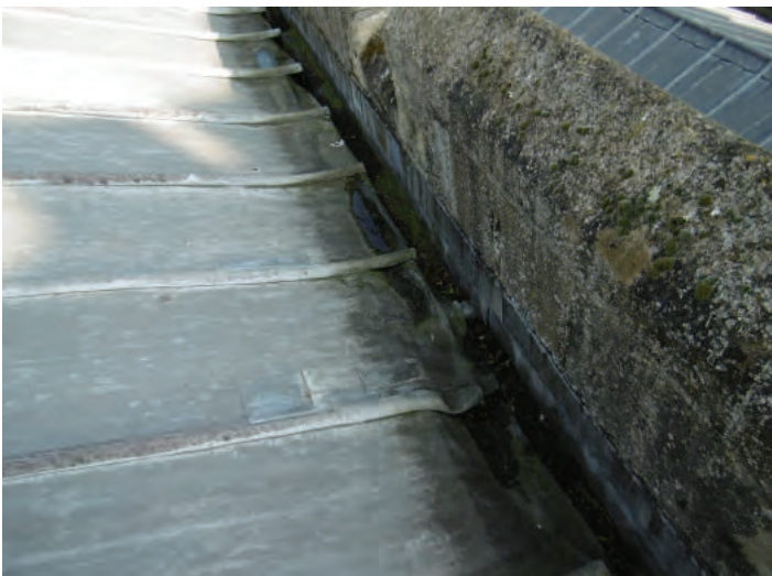
LEAD CREEP ON THE NAVE ROOF
