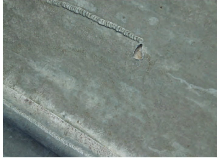
THE LEAD CORROSION ON THE NAVE ROOF
