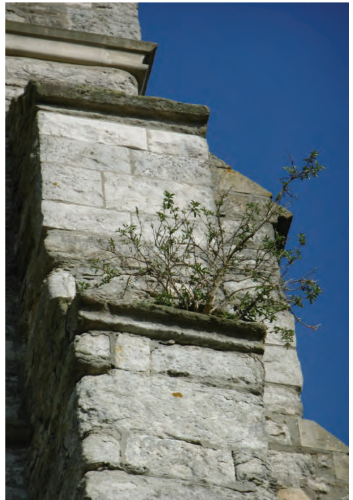
VEGETATION GROWTH ON THE TOWER
