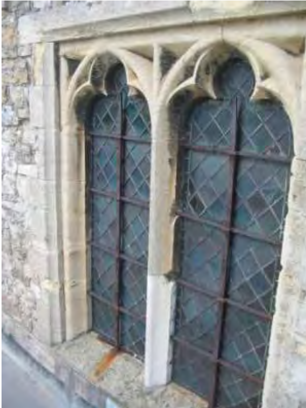
Rusting Ferramenta to South Nave Clerestory
